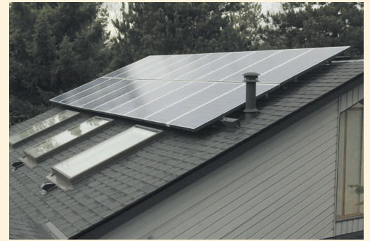
The 18 roof-mounted Sharp polycrystalline panels on the Baasch home are invisible from the street.
