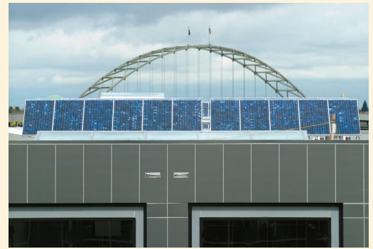
Polycrystalline roof-mounted solar panels are part of the 22.4-kilowatt system installed on Brewery Blocks Building 4.
