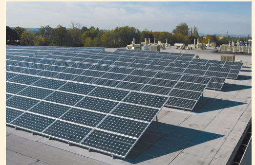
The 616 Sharp solar panels mounted on the Kettle Foods roof will produce approximately 120,000 kilowatt hours of electricity each year. The solar installation is the largest in the Northwest.
