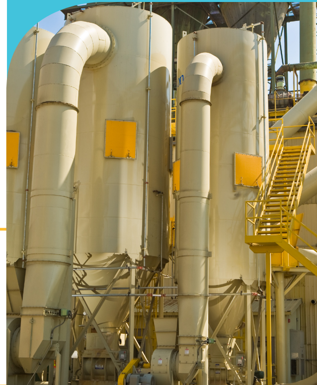
Sawmill baghouses (dust collectors)
