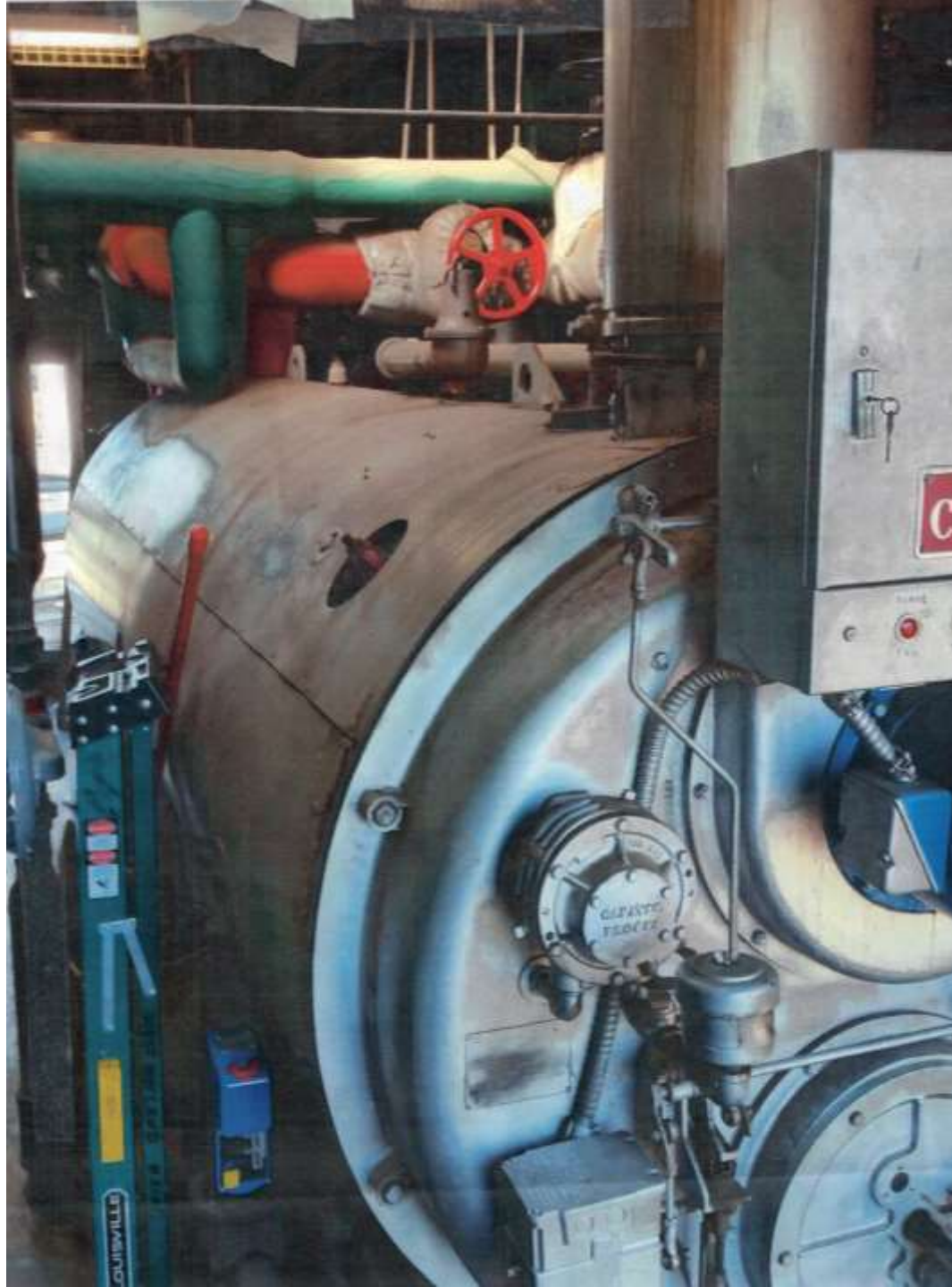
1 of 2 Original Gas-Fired Boilers (Fed by 5inch Nat Gas Line @ 5 psf)
