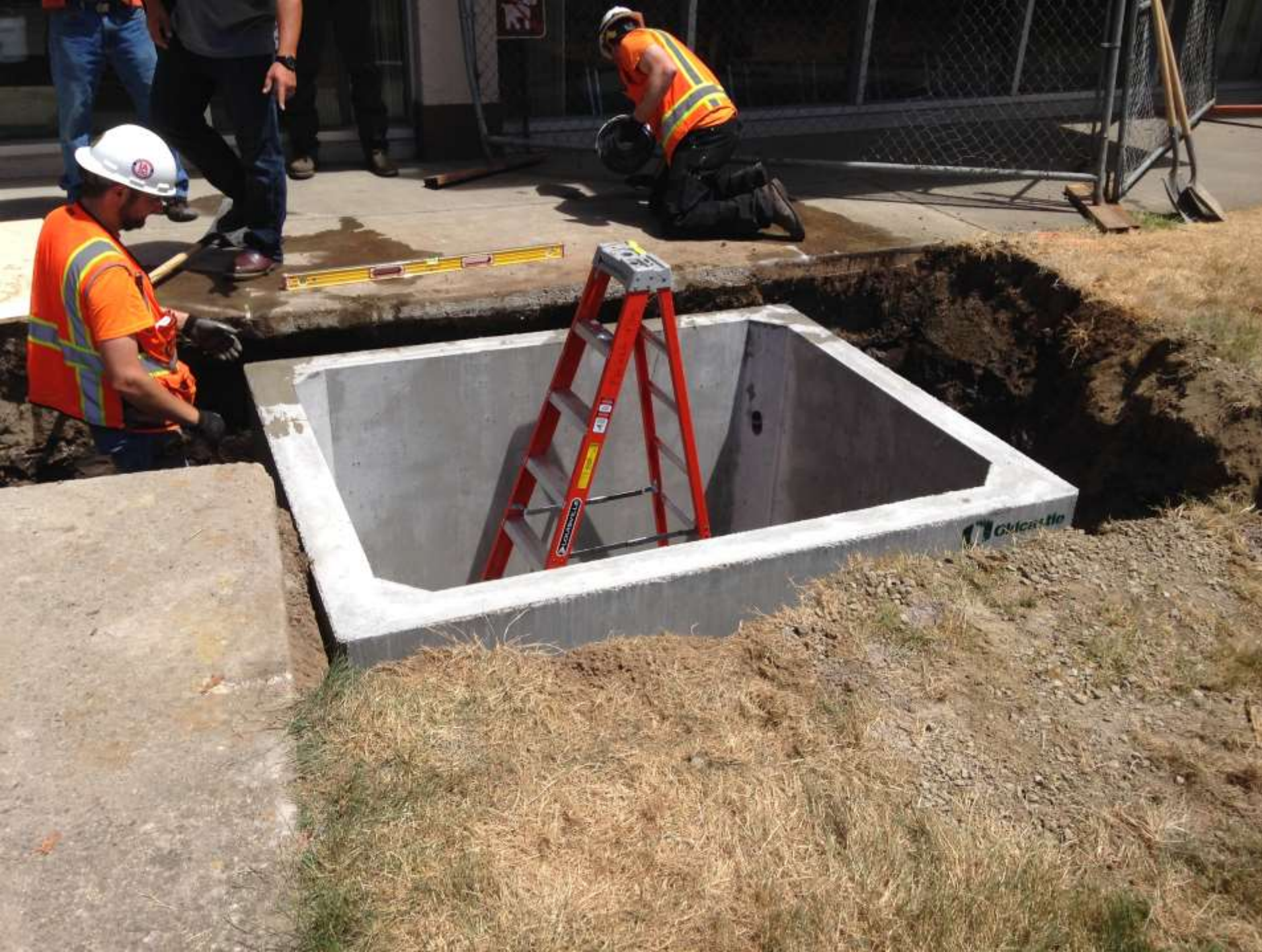
New Dom Water DCVA (Double- Check) Vault
