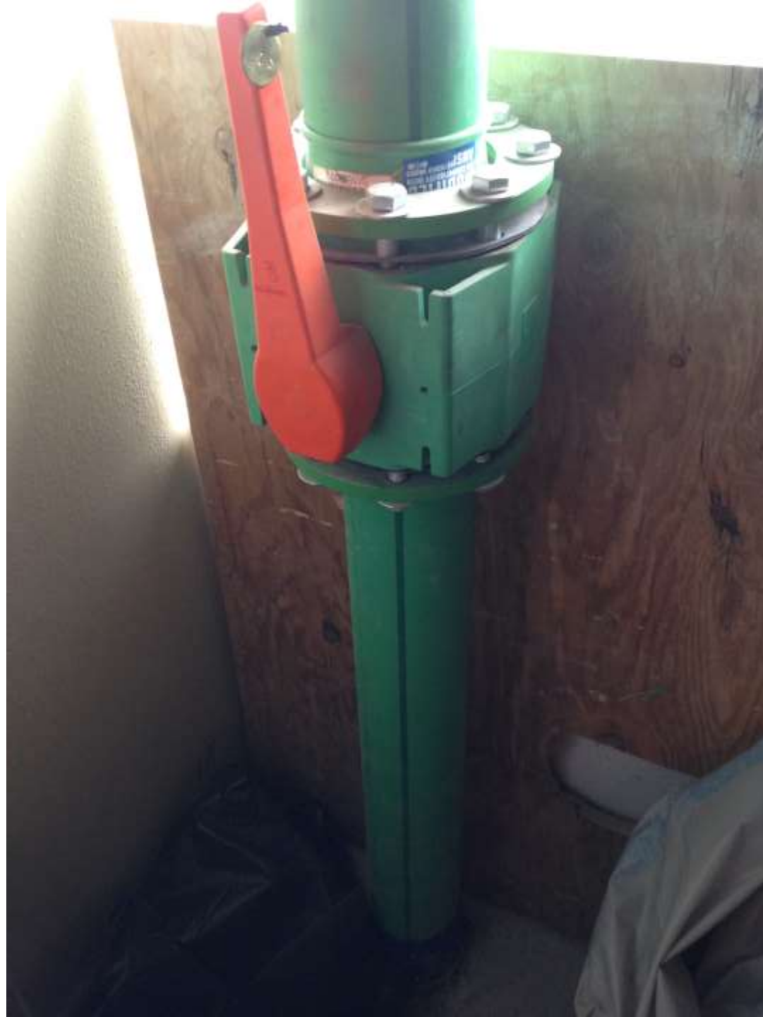
Domestic water shut-off
