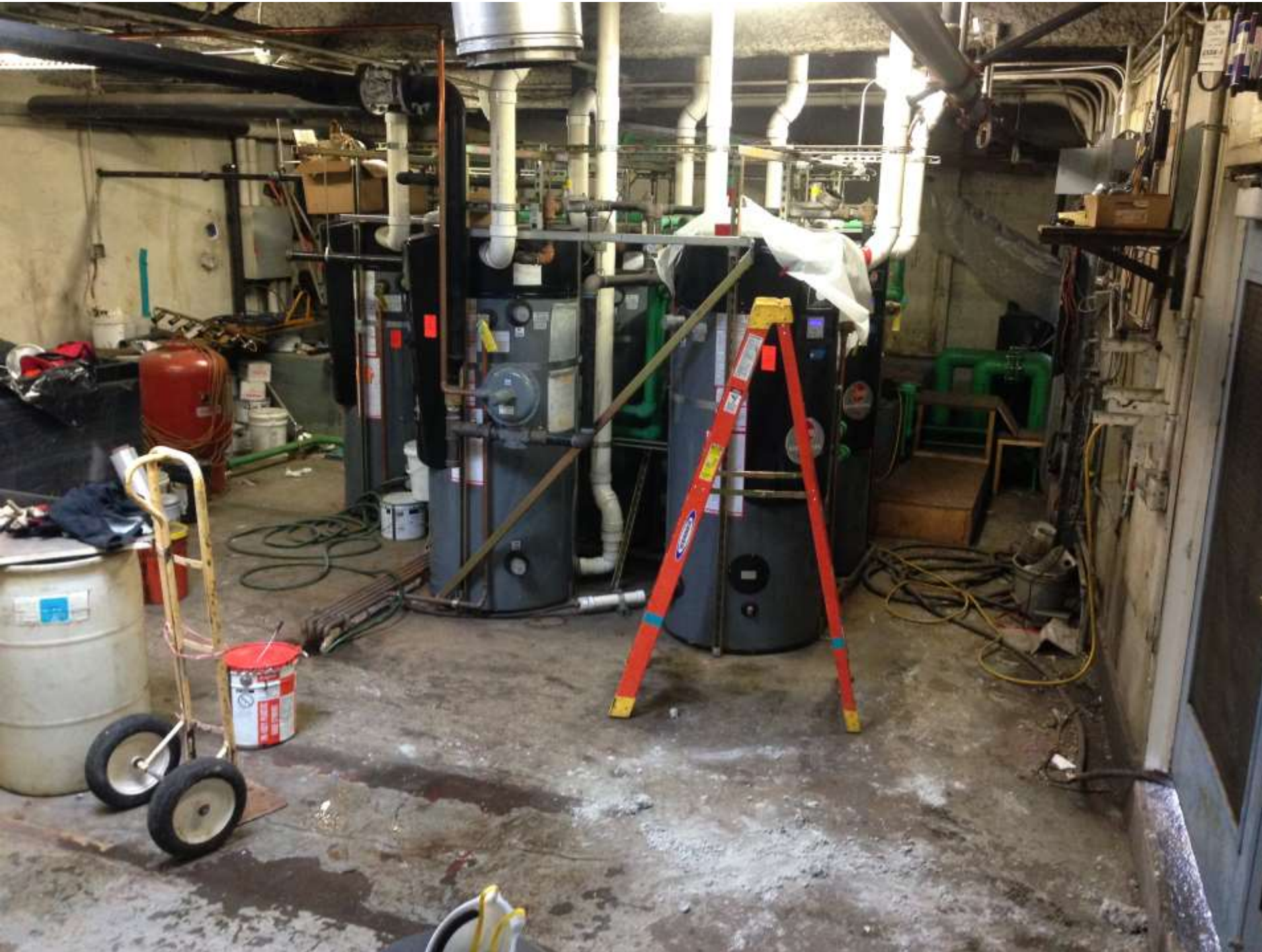
Boiler combustion/ exhaust ducting in place
