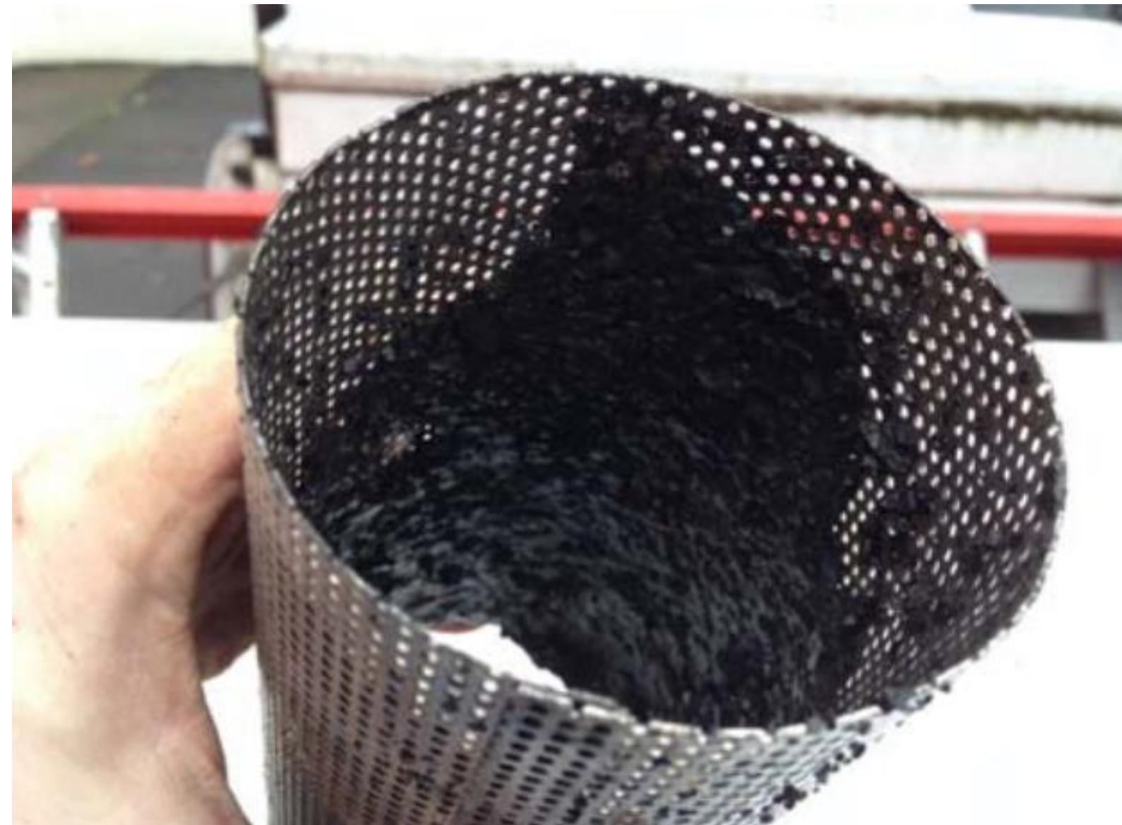
Lack of Equipment Maintenance
