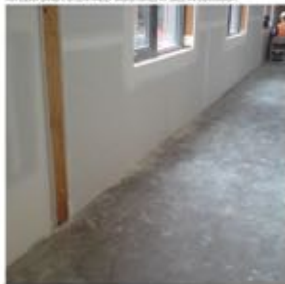
AIR LEAK (AND POTENTIALLY MOISTURE) AT SLS IN CORRIDOR
