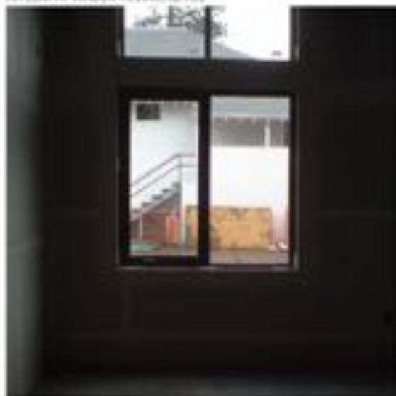
AIR LEAK AT WINDOW IN MIMERSPACE
