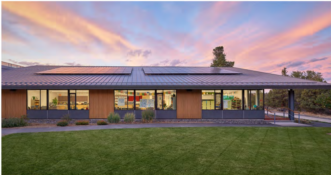
24.6-kW solar panel array at Cascades Academy of Central Oregon
