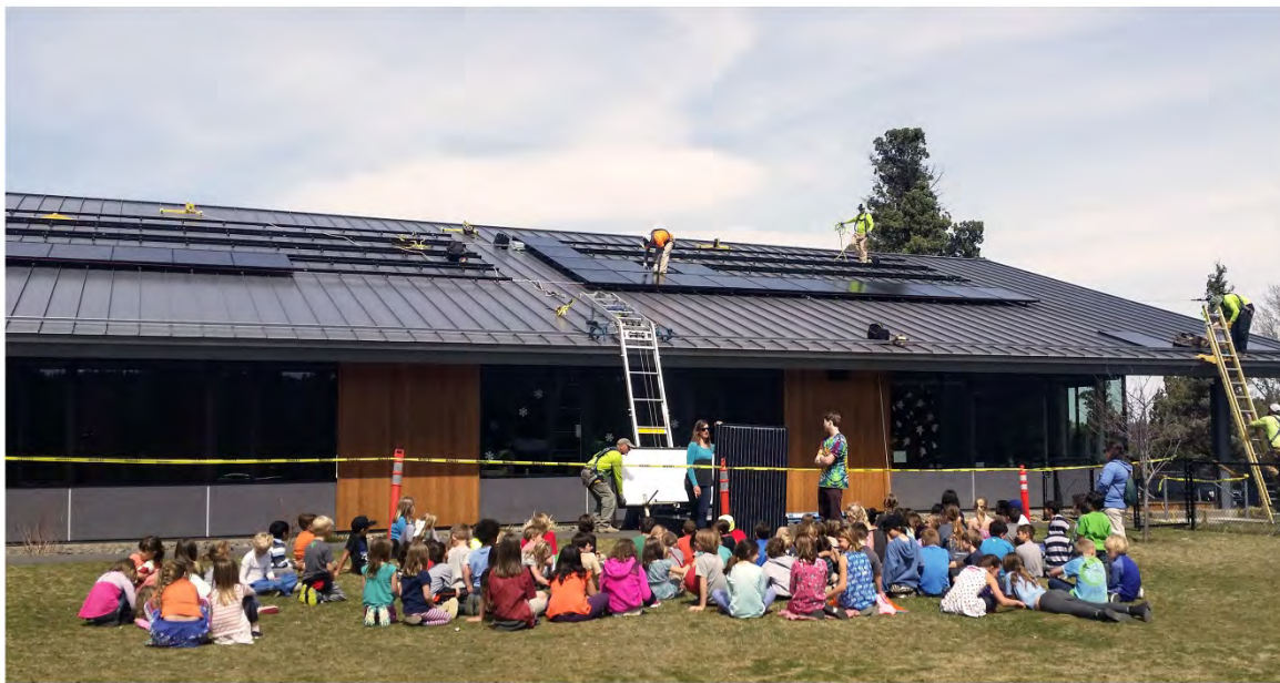
Students watch as solar panels are installed at Cascades Academy of Central Oregon
