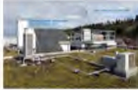
New air-side heat recovery and energy recovery ventilation (ERV) units
