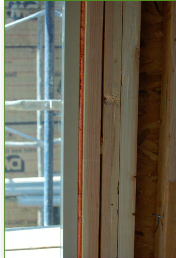
Photo courtesy of Ken Baker, K energy
