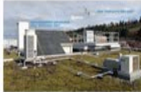
New air-source heat recovery and energy recovery ventilation (ERV) units
