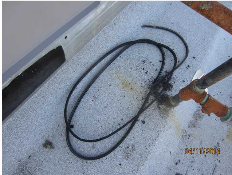
Figure 8. Poor Maintenance Practices
