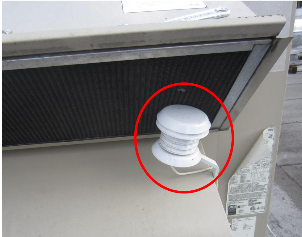
Figure 19. Outside Air Temperature and Relative Humidity Sensor
