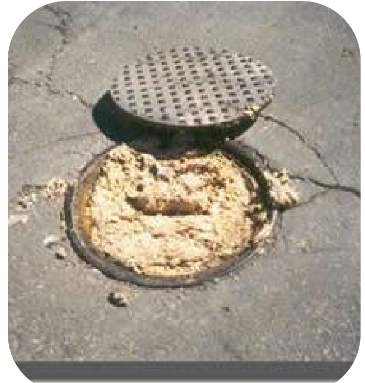
Brown grease (FOG) clogging a sewer line.
