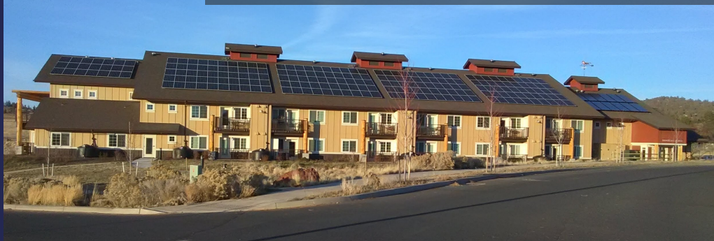
IronHorse Lodge 64 kW Solar PV
